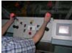
Dead man switches ensure operator safety
